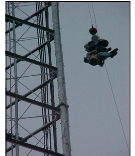
A tower climber is hoisted into position near the top of the tower.
